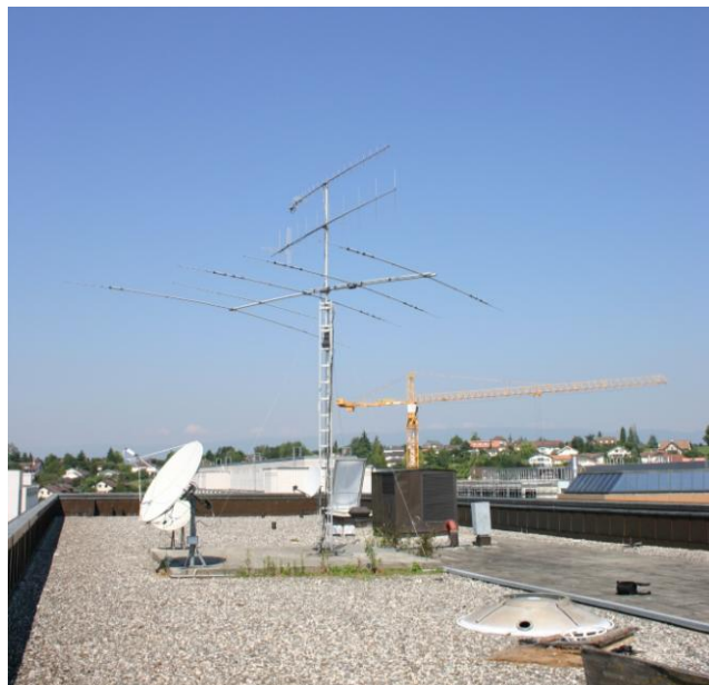
Figure 2: Current installation on the roof of the EL building.
