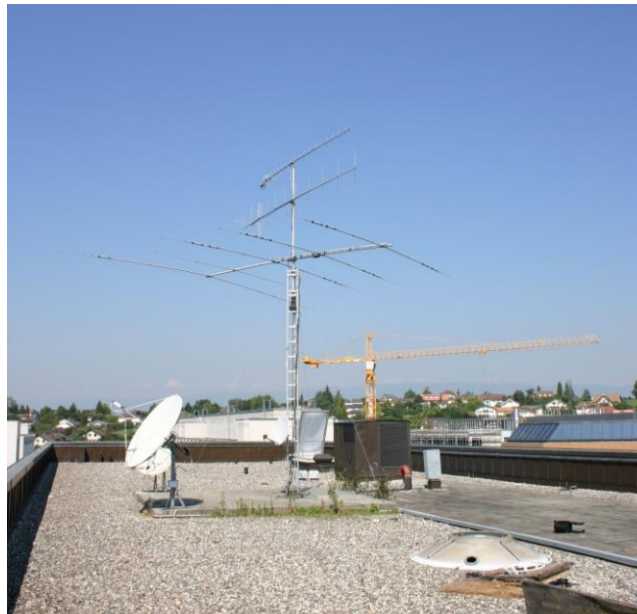
Figure 11: Current installation on the roof of the EL building.
