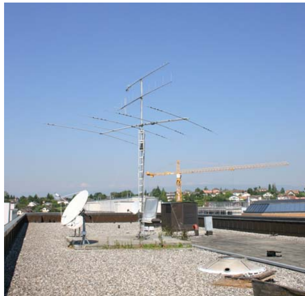
Figure V-3: Current installation on the roof of the EL building.
